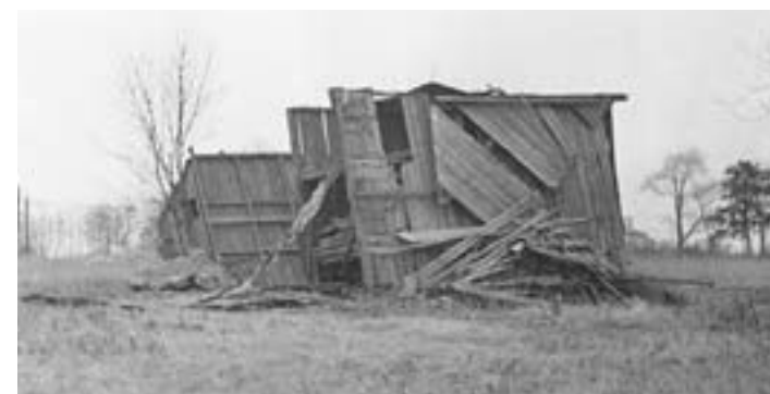
The remains of Cyrus Eli Perry's Ventilated Tobacco Barn, near River Road and Willard Avenue.
